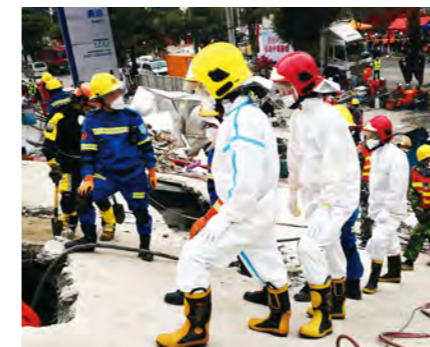
△ Quanzhou Petrochemical emergency base participates in the rescue of the "3.7" collapse of Xinjia Hotel in Quanzhou
